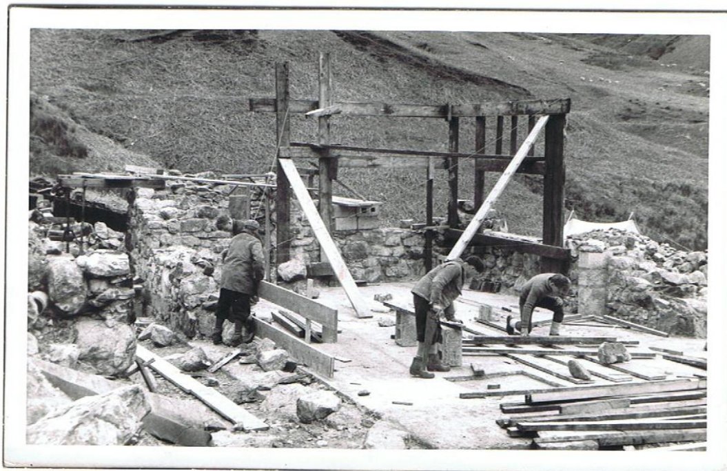
The Kitchen Wall of Bryn Hafod going up – submitted by Nick Smyth
